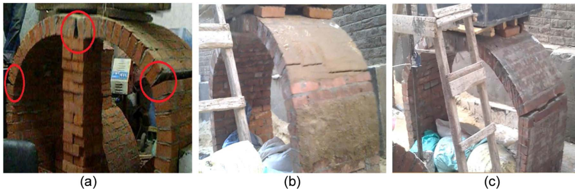
Fig. 9. Failure of masonry vaults a) unstrengthened, b) vaults strengthened by polyester mortar and c) vaults strengthened by GFRP.
